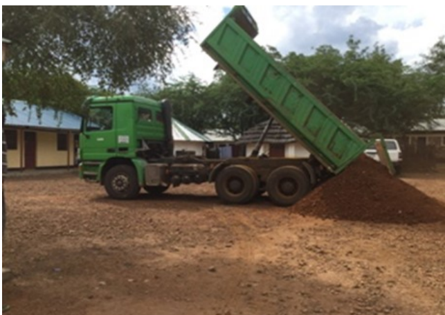
Work in the compound after the flood
